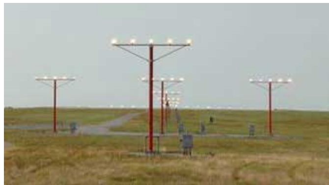
Figure 2. A MALSR Showing the 1000-ft Station Crossbar
